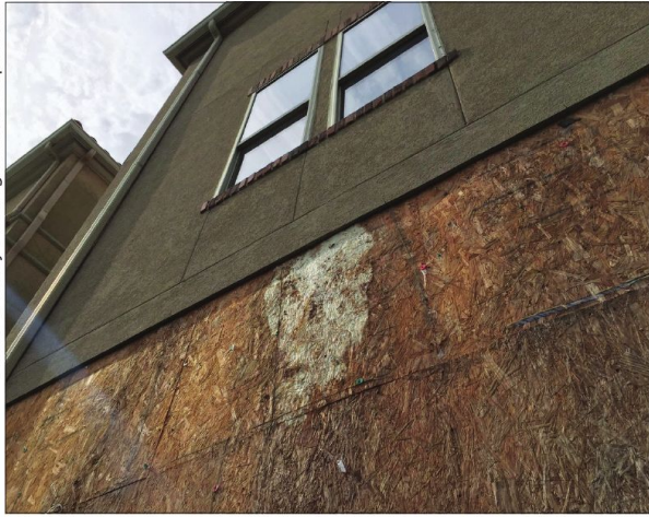
Moisture damage on wood frame low-rise building.
