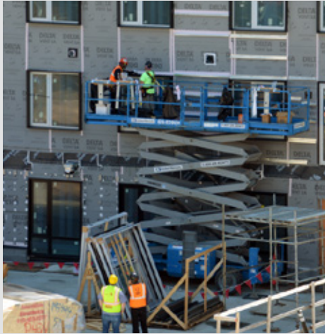
The team installing DELTA®-MULTI BAND 100, a versatile tape with very strong adhesion
